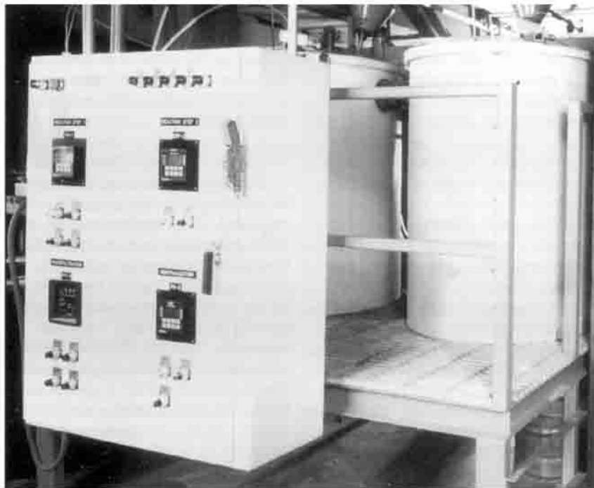
Figure 2. Water-treatment unit relies on both pH and ORP controllers.
